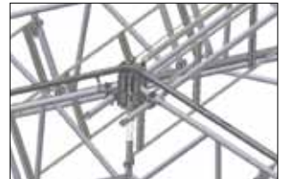
The fall protection anchor in place
